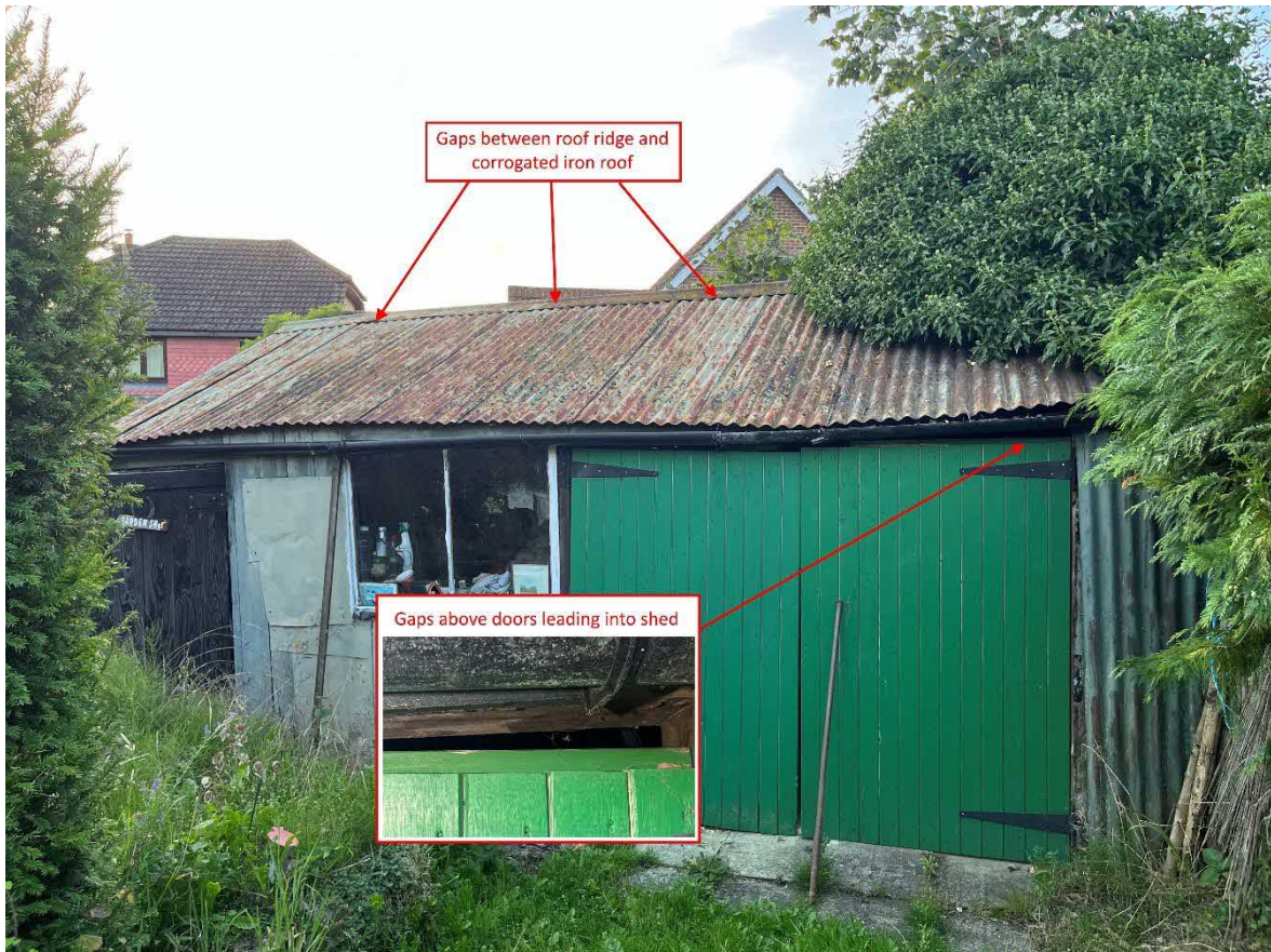
Image 4.3.2.2. Location of bat access points on the south elevation of the Outbuilding.
