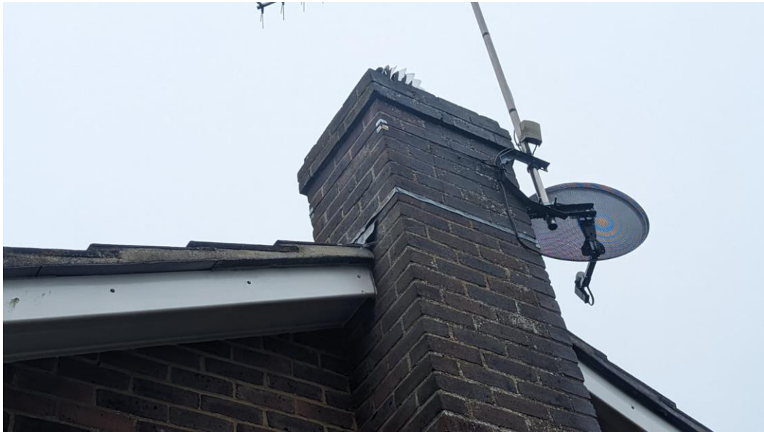
Photo 10 – Chimney with lifted flashing
