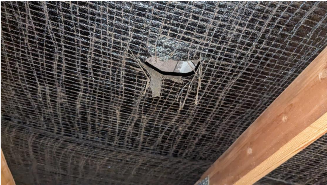
Photo 4 – Internal loft void, torn felt
