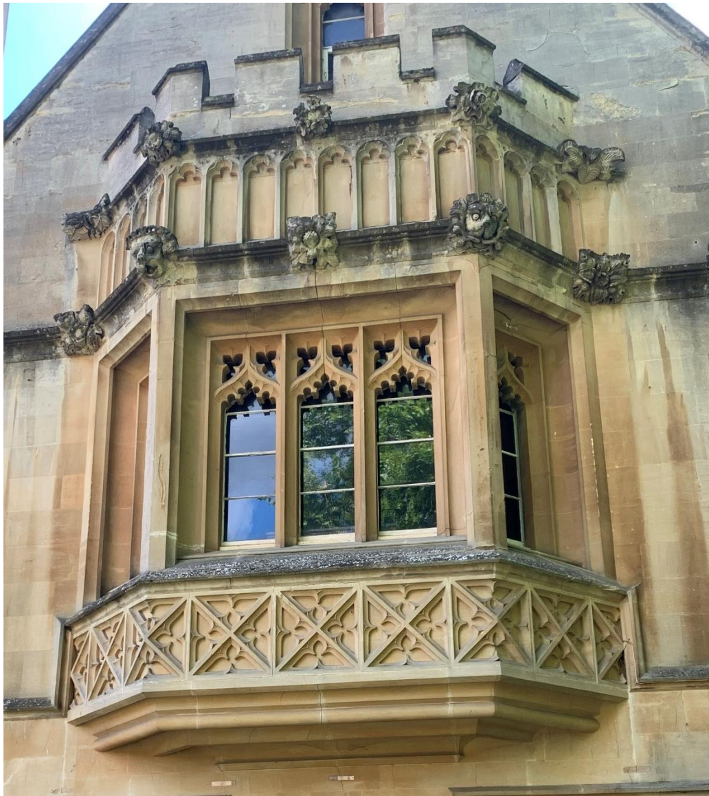
Oriel window on northern elevation of the Cloister lighting the Old Library
