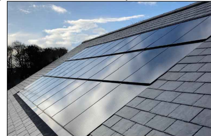
PANELS TO BE 'IN-ROOF' MOUNTED TO SIT WITH PLANE OF ADJACENT AREAS OF ROOF SLATING AS ILLUSTRATED ABOVE.
