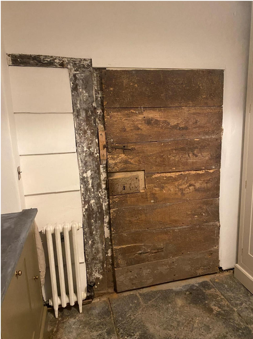
Image 1 – Photograph of rear area of larder (GF3), demonstrating use of existing post within wall to left of doorway, and no freestanding post has been installed.
