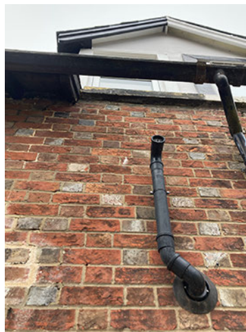
Image 12 – Subsequently installed boiler flue with additional parts
