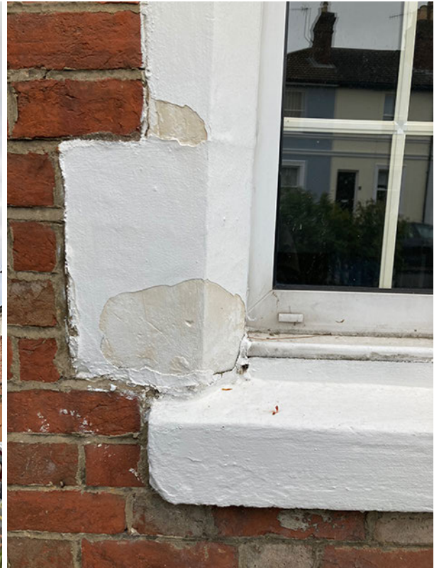
Image 07 – Evidence of cracked, flaking paint
