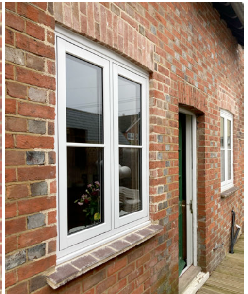
Image 14 – New kitchen window reveal in the foreground – now all three apertures have curved soldier brick lintels
