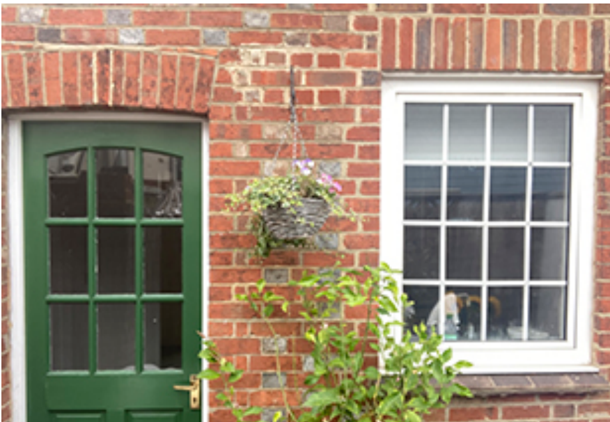
Image 13 – Existing kitchen window with non-original straight soldier brick lintel (now replaced), adjacent to back door with original curved soldier brick lintel
