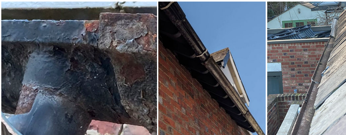
Image 01 – Close up shows corrosion to existing cast iron goods
