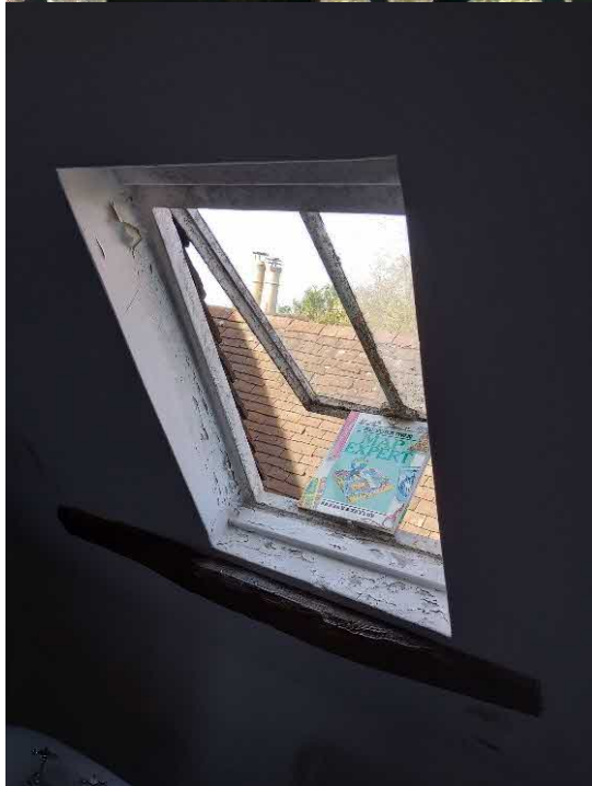
Window 19: gap between opening light & frame
