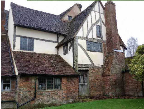
North-west elevation catslide and kitchen window range. North-west elevation projecting West end range.
