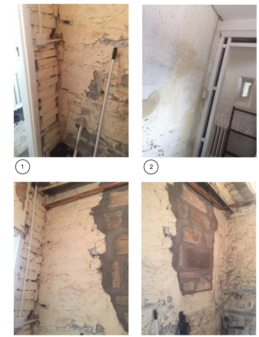
Existing Internal Photos Existing internal walls to be removed - no loss of listed fabric of any significance
