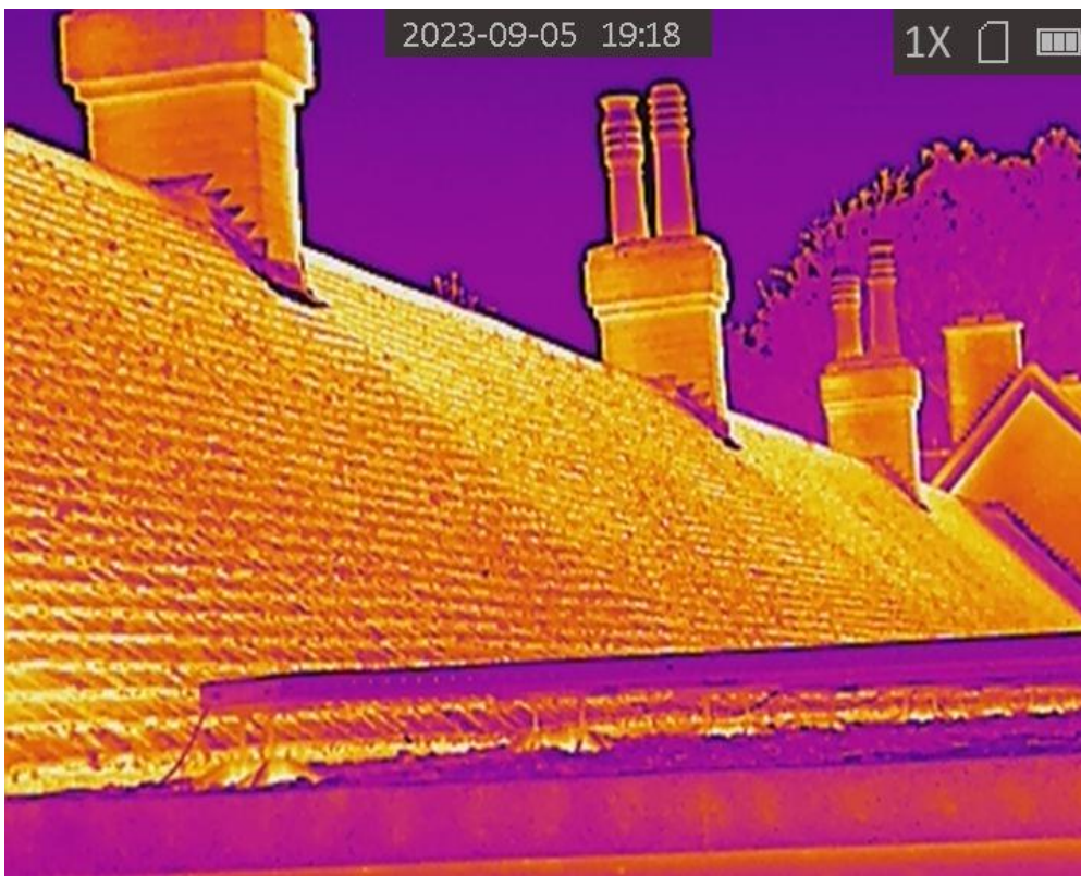
Photograph 12: Thermal camera field of vision on 05/09/2023.
