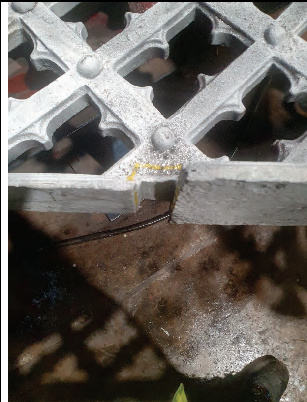
Photograph 9, indicating fracture to spandrel haunch at the location where section properties curtail abruptly likely a stress concentration.
