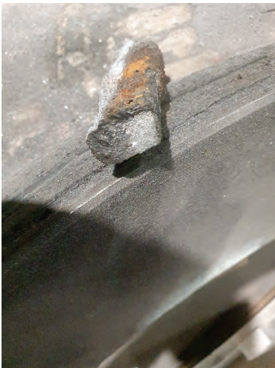
Photograph 8, extracted section of keystone that had fused with the locating groove, note the shiny fracture surface perhaps an indication graphitic corrosion.
