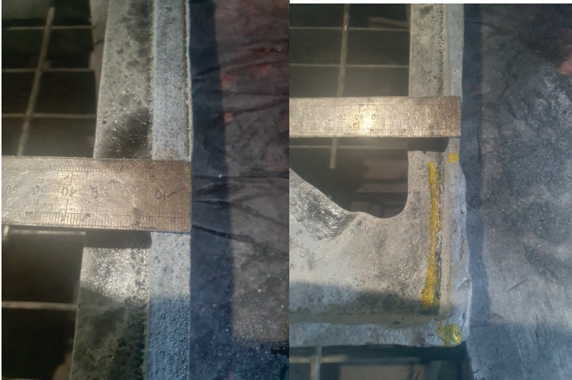
Photograph 14 & 15, indicating the balustrade infill panel at its junction with standard. Note the necing of the section left (no necking approx. 12mm) and right (necking 7mm).
