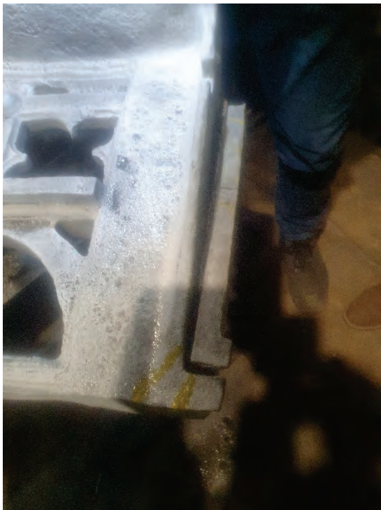
Photograph 6, indicating fracture to key stone (voussoir) bottom note the residual key stone component had not become free from the grit blasting preparation. This was investigated and it was found that the keystone section was extensively corroded, seized and partly fused into the groove in which it locates. CIWS operative managed to carefully tap this out with mallet and chisel exposing the original casting groove.
