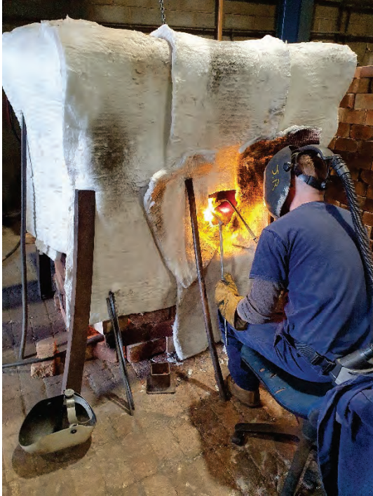
Photograph 2, indicating fusion welding process where component is locally heated and insulated then welded with oxyacetylene touch electrode and flux. CIWS noted the important of matching the grade of cast iron the parent metal metallurgy which is informed by sampling in their yard.
