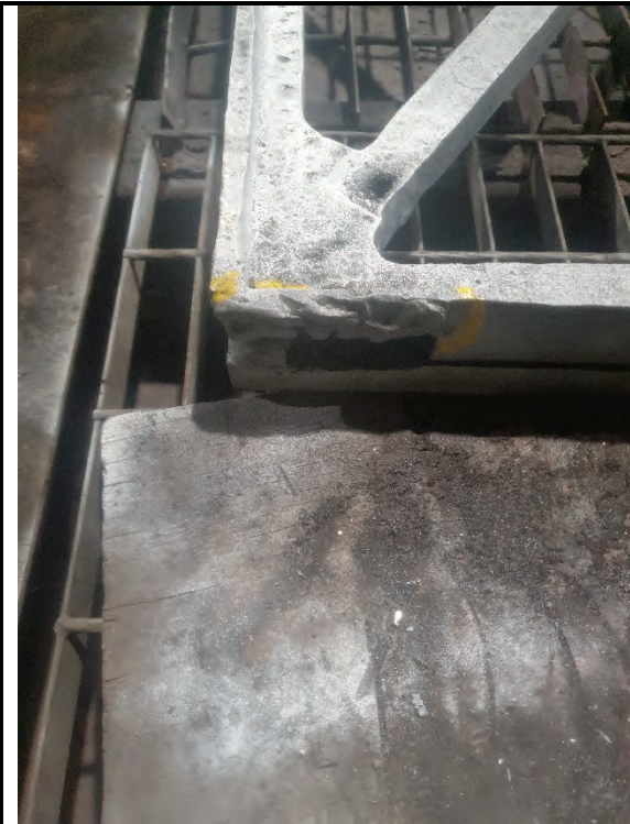
Photograph 13, indicating bottom corner of balustrade infill, note historical in situ attempts have been made to weld the panel forming an ad hoc repair. Weld quality was of poor quality. It is likely this was done to counter the balustrade panel joints which are generally reported to open up.
