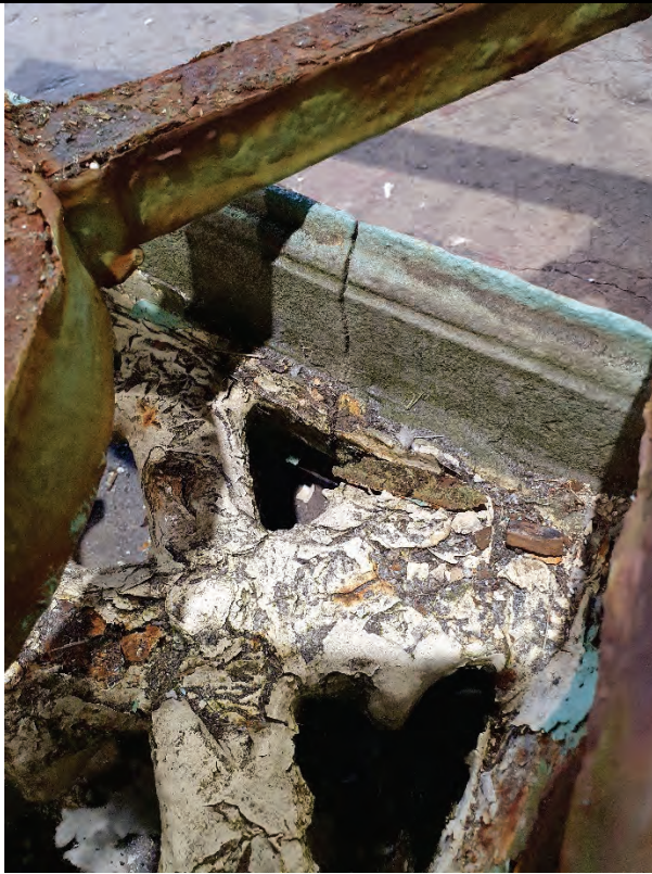
Photograph 11, indicating 2 nd spandrel half which had not been grit blasted at the time of the visit though a significant full depth fracture was noted to the haunch propagating full depth through the entire shoulder of the spandrel. No bolt holes in the vicinity of the fracture.
