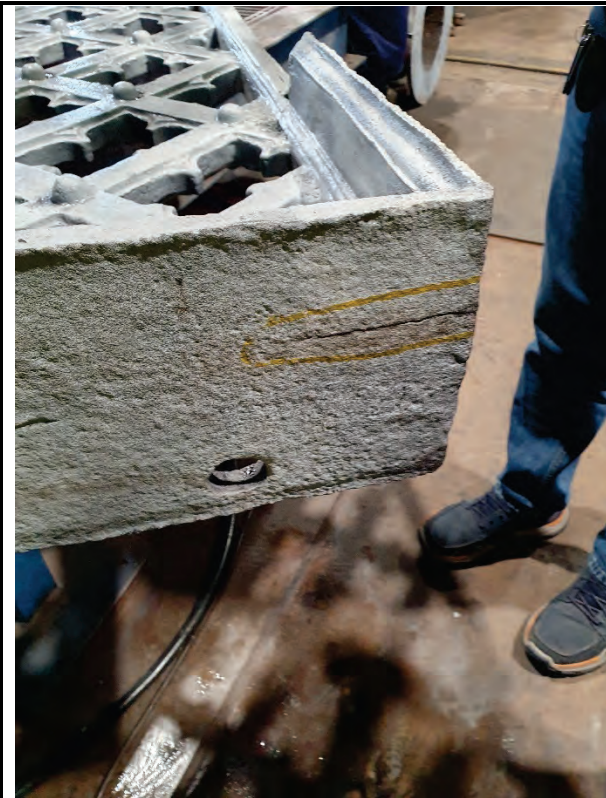
Photograph 5 indicating fracture to spandrel haunch zone note does not initiate or propagate to a bolt hole.
