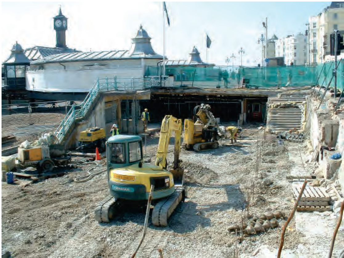
Photograph 1 - Indication the Aquarium Colonnade frontage immediately east of Brighton Palace Pier circa 2001 during reconstruction. Note original sea wall right of frame with associate steps and more modern on current southern sea frontage alignment steps left of frame.
