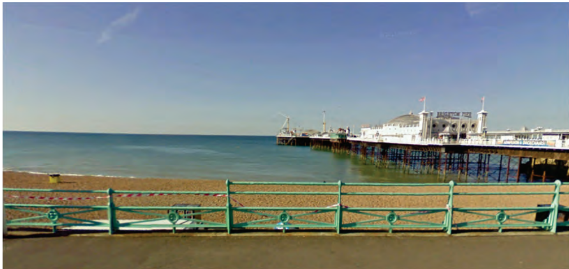
Photograph 2 - indicating Junction of Seafront railings at the Aquarium Colonnade. Left are the original seafront railings, right extended railings adopting similar detailing and connections, baseplate connection concealed.
