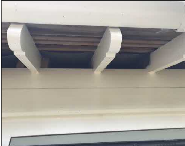
Image 7: The eaves around the northern wing are open, providing access to any voids present.
