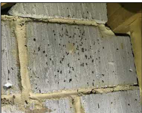
Image 11: Bat droppings were found on a block gable end leading north. This image is from 2022 but a similar amount was found in 2023.
