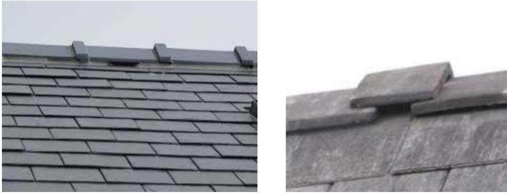
Figure 10: Examples of ridge tile access.
