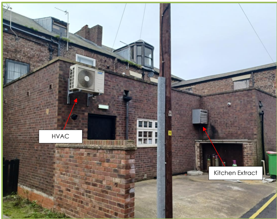
Photograph 1: Identified Building Services Plant associated with 'The Manor Bar'
