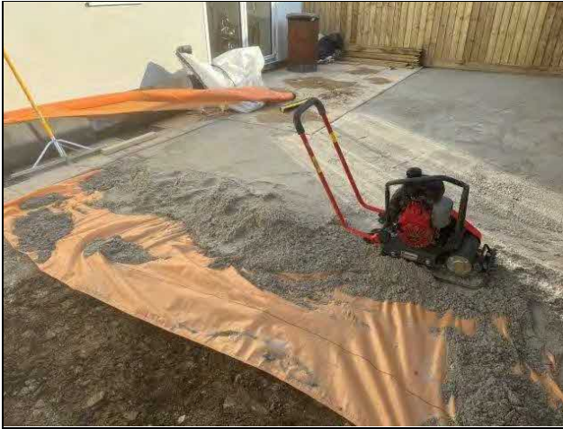
Plate 17: View showing sand blinding laid over additional membrane in garden area in preparation for astroturf
