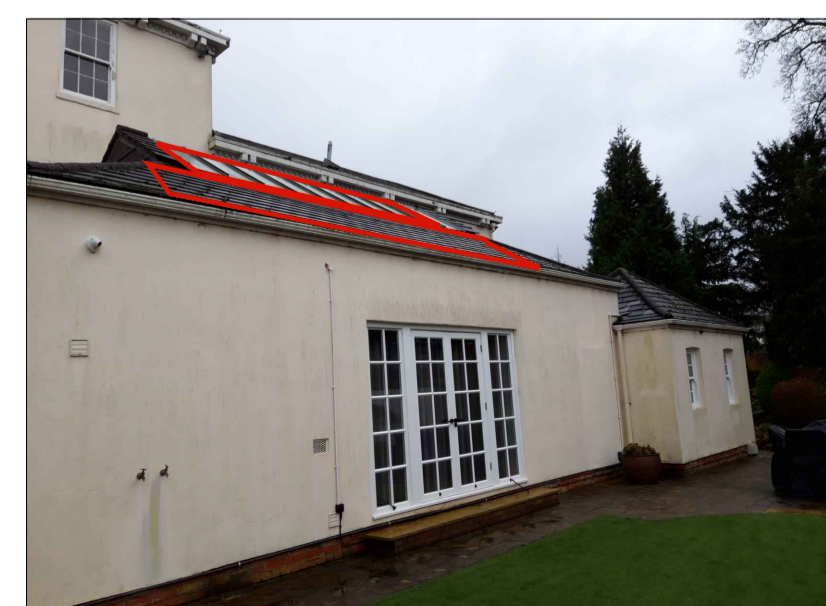
Photo of Elevation with Solar Panels
