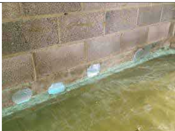
SAGM patches applied prior to inspection to the perimeter membrane within Plot 10.
