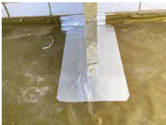
Plot 3 retro fit detail over the damaged membrane that is under the internal block work wall.
