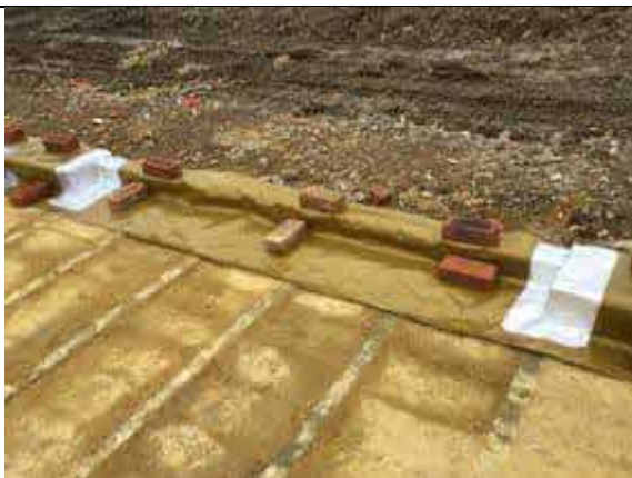
Plot 6 typical door threshold seal using SAGM.
