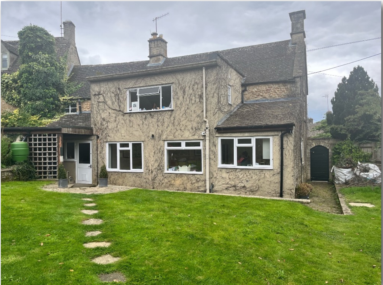
The above photograph shows the rear (East) elevation of the existing cottage, clearly showing the existing previous rendered extension.
