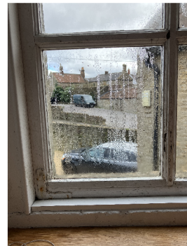
WF.01 bottom rail to lower opening casement has rusting metal angle repair and two sections of moulded glazing bar have been replaced with square section
