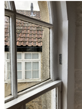
WF.01 meeting rail to upper fixed casement sections of moulded glazing bars have been replaced with squared sections
