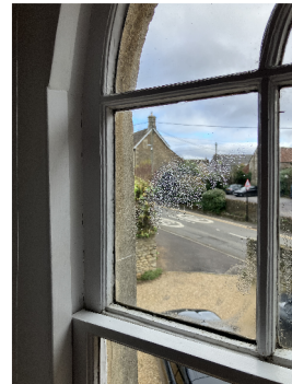
WF.01 meeting rail to upper fixed casement sections of moulded glazing bars have been replaced with squared sections
