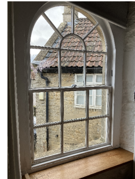
WF.01 bottom rail to lower opening casement has rusting metal angle repair
