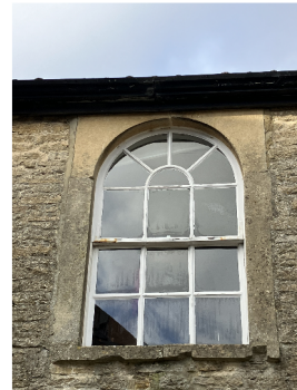
WF.01 meeting rail to upper fixed casement has rusting metal angle repairs
