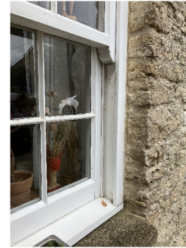
WG.02 sill and outer lining to frame show signs of deterioration
