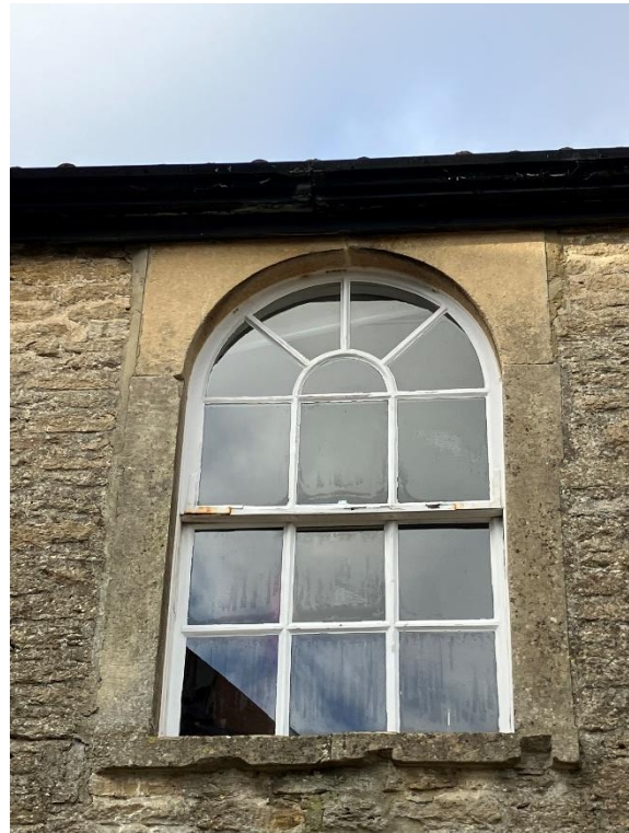
Fig. C.2 First floor courtyard window – exterior showing rusting angle repairs
