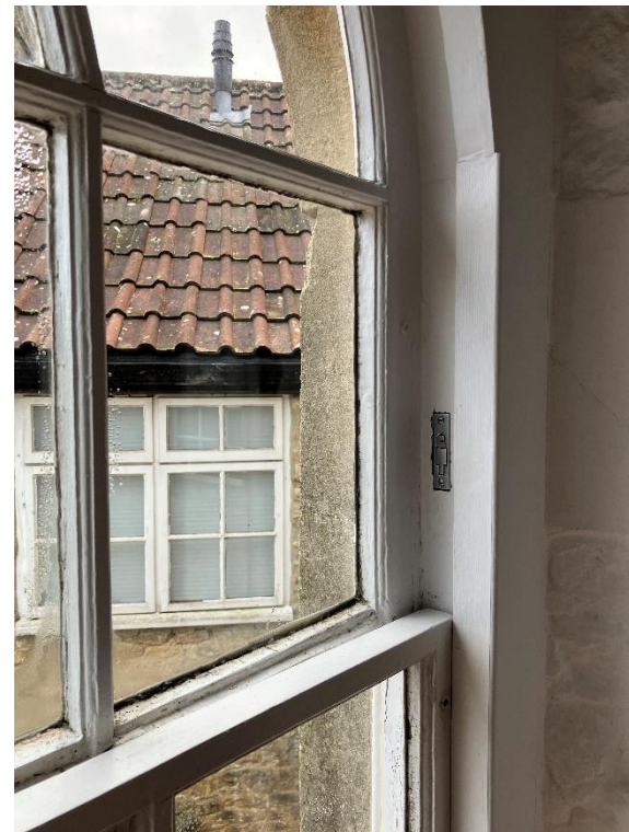
Fig. C.4 Detail at meeting rails, shows repairs to upper casement meeting rail, moulded detail lost
