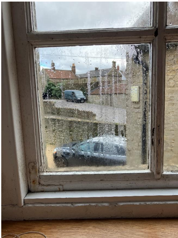
Fig. C.3 Detail of metal angle repair, moulding along bottom rail have been lost through repair
