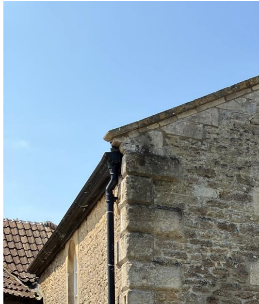
Fig.4 Clipped eaves with fascia board, courtyard elevation, same detail to roadside elevation
