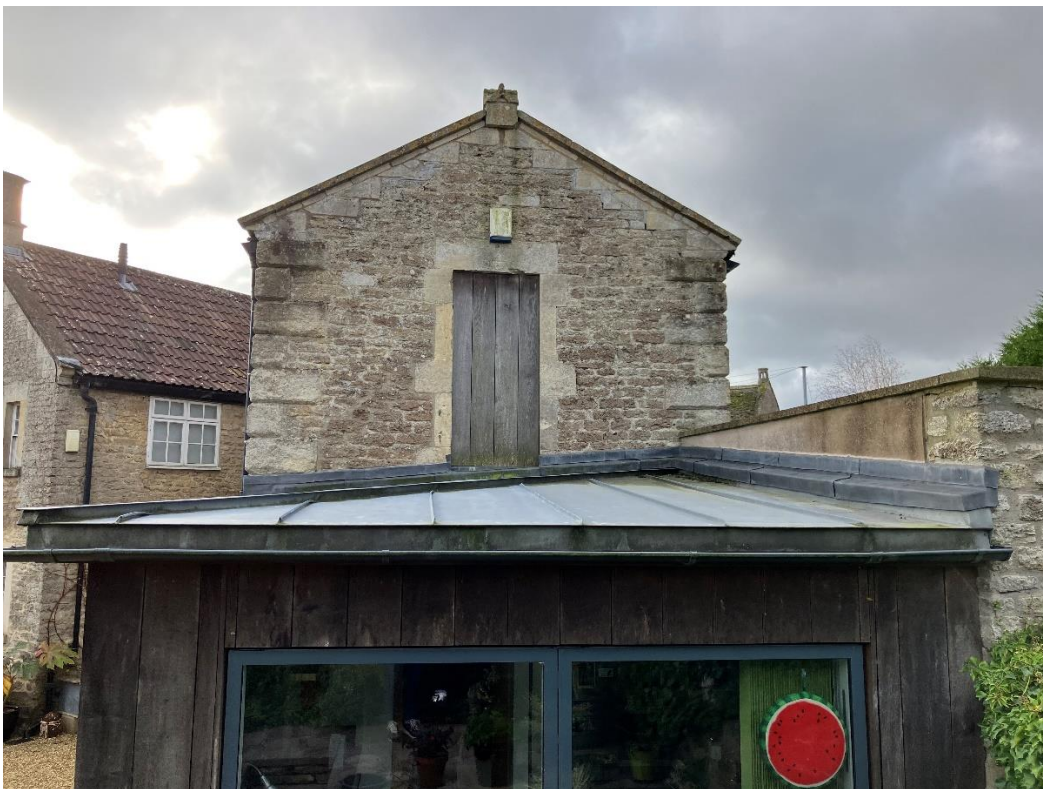
Fig.5 Zinc roof, shallow pitch with deep overhang at eaves and stepped lead detail at abutments with the existing stone gable and stone/render wall to roadside.
