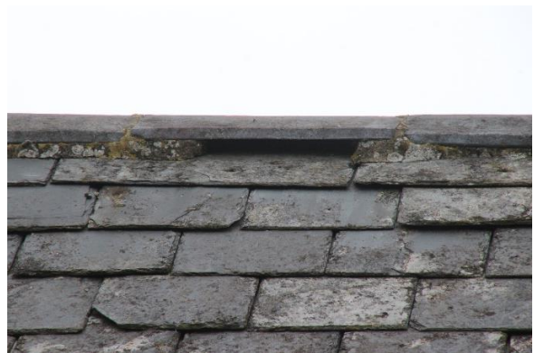
4. Gaps under ridge tile
