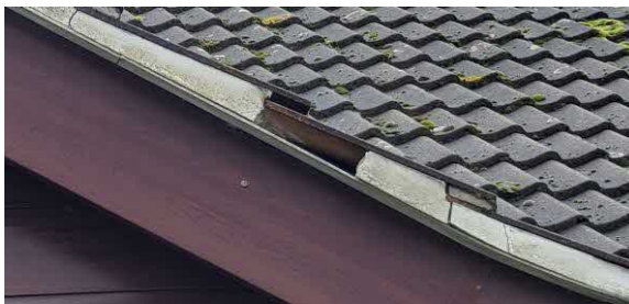
5 Example missing mortar from rake
