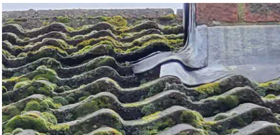
7 Gap between tiles and lead flashing
