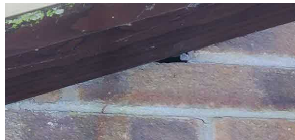
8 Example gap under eaves
