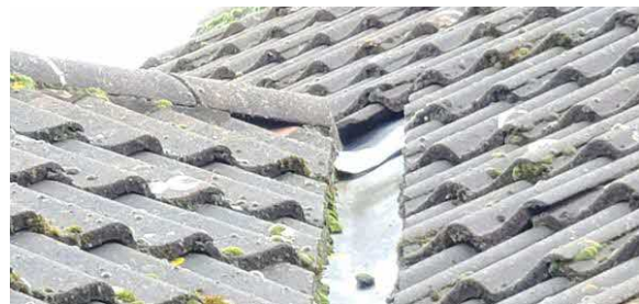
6 Missing mortar from ridge, and gap under tiles at valley
