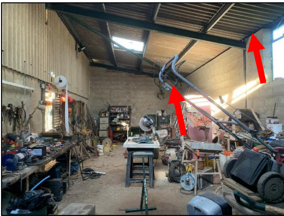
Figure 5. Internal of lean-to – red arrows indicate access points to cavities within the block walls
