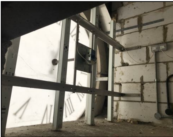
Image 12: View of loft void two. High light ingress from translucent clock face.
