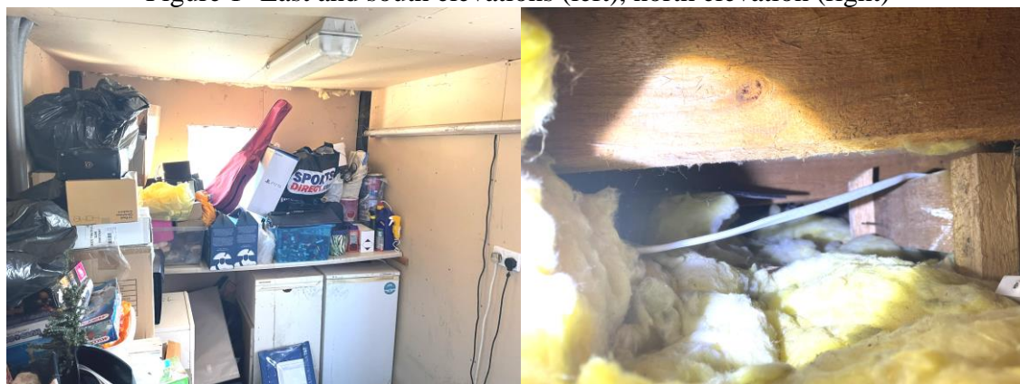
Figure 2- Internal view of extension (left) and void beneath the flat roof (right)
