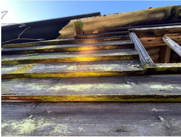
Photo 7: Eastern weatherboarded gable end, with no gaps beneath weatherboarding or around window frame
