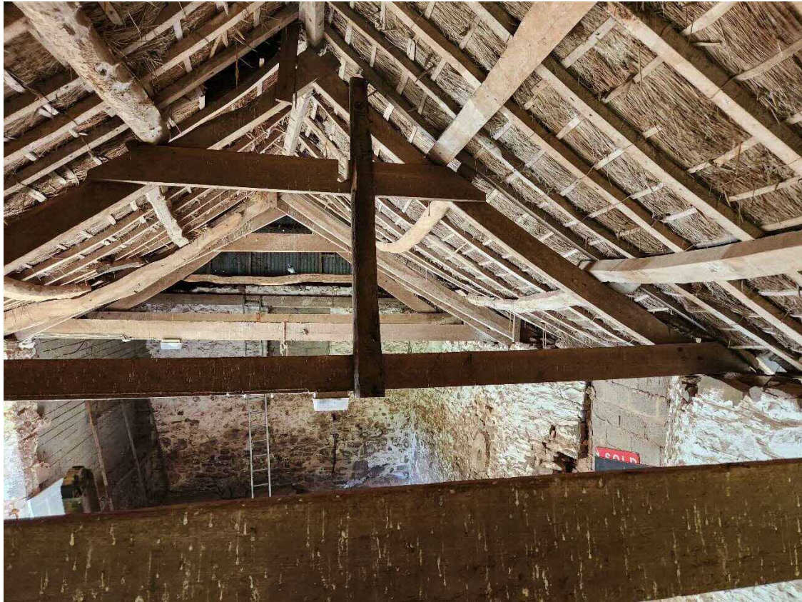
Above: Over clad thatch roof supported on cut rafters, purlins and trusses.
