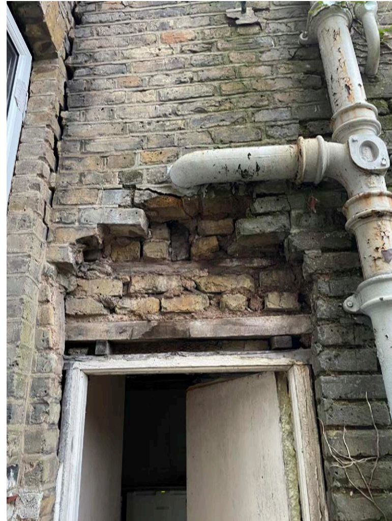
Missing brickwork to the existing garden door is dangerous and reinforces the need to rebuild the annex before the property can be extended.
