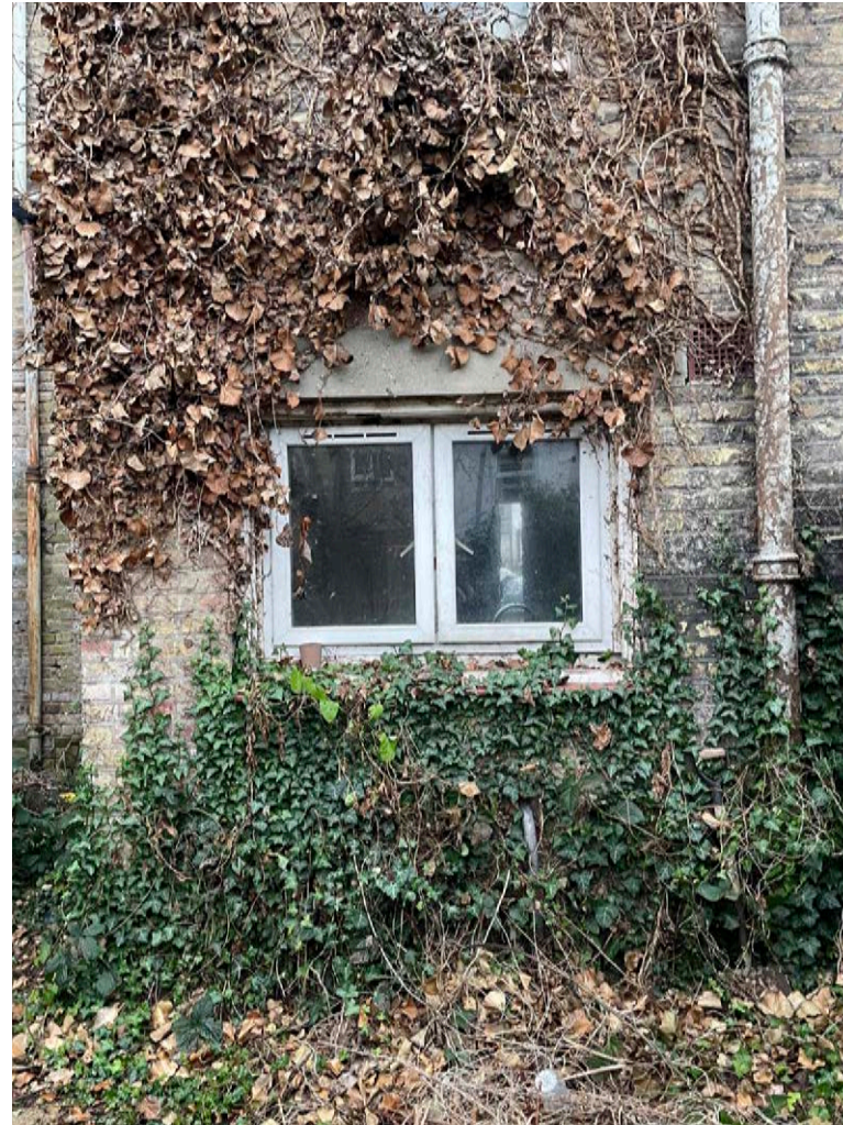
The existing rear of the house is in poor condition with vegetation covering much of the annex. The rear annex is also in a structurally precarious condition with cracked and missing brickwork. No original windows survive.
