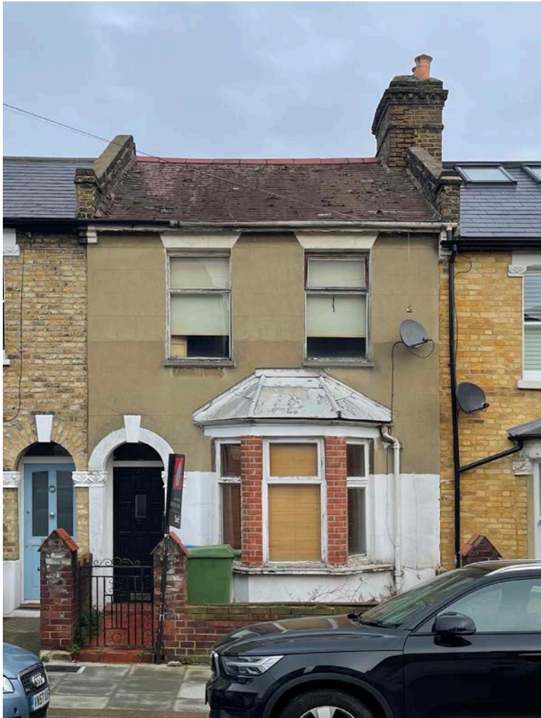
The front of the house has been rendered in cement render, covering the original brickwork. The bay has been remodelled in the past with red brick and a steel roof. The original slate roof has been coated in a red bituminous paint. Design and Access Statement - 27 Goodrich Road, SE22 9EQ
