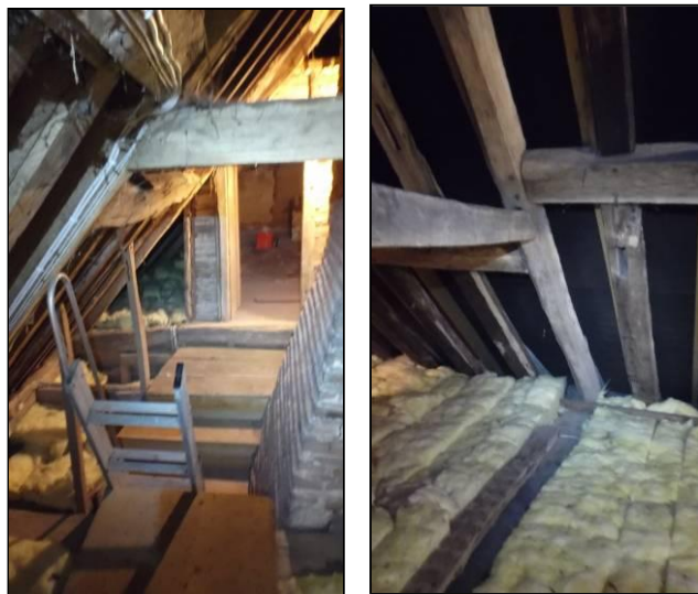
The two end assemblies on Truss C, looking north (right) and north-east (far right). Note the redundant mortice on the re-used timber employed as a rafter on the far right.
