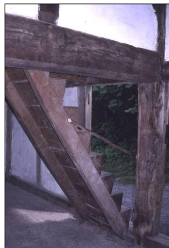
A typical ladder stair of the type that may have been employed at South Mundham House.
