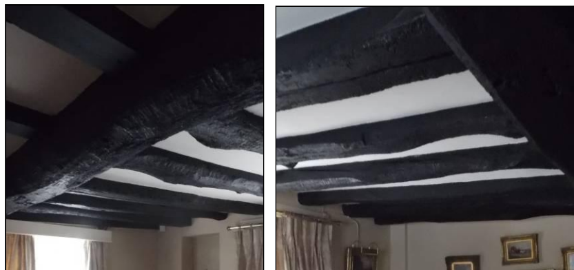
The floor beam and joists, looking south-west (above left) and looking north-west (above right).
