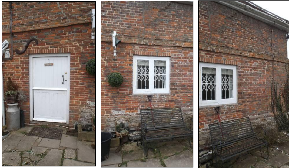
The inserted door opening with stable door (above left); the original window opening (above centre); and the partially re-built wall to the north-west corner (above right).
