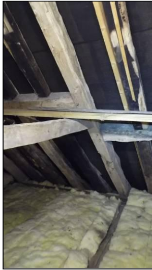
The two end assemblies on Truss D, looking north (far left) and north-east (left).
