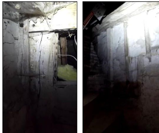
Timber-framed elements in and adjacent to the west wall (right and far right).
