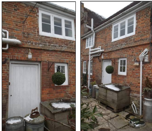
The inserted window and door openings at ground level and the two first floor windows above them (right and far right).
