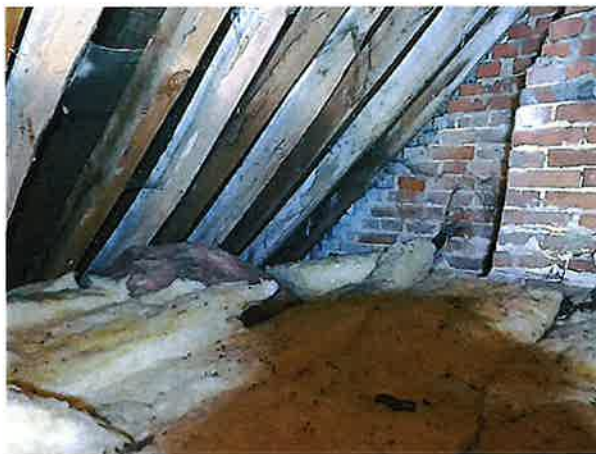
Scattered bat dropping on insulation material in roof void of SW annexe
