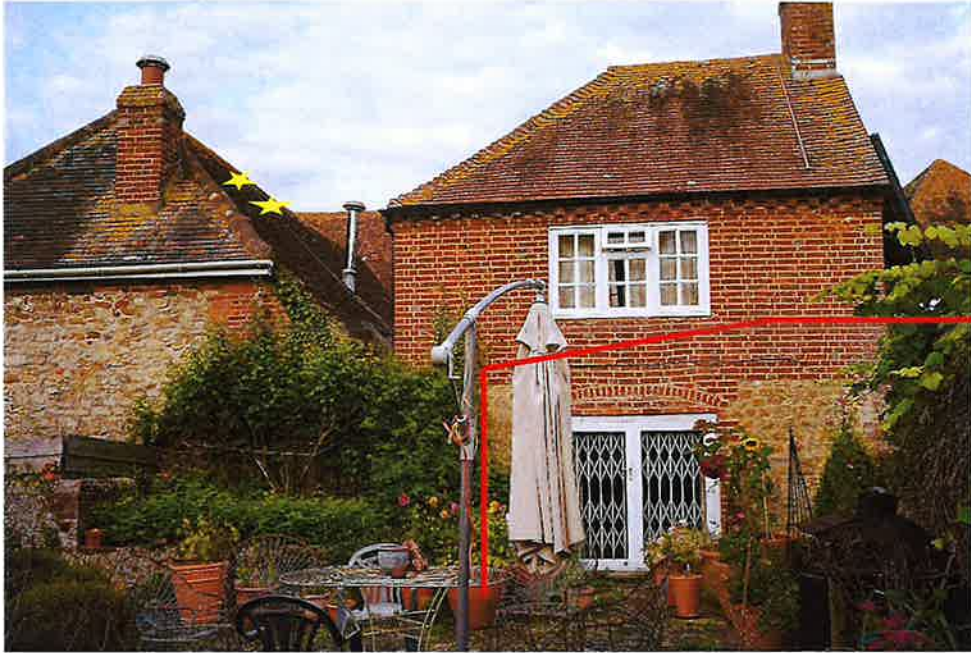
Approximate position of proposed new roof lights (starred) & approx. position of proposed extension (red line)
