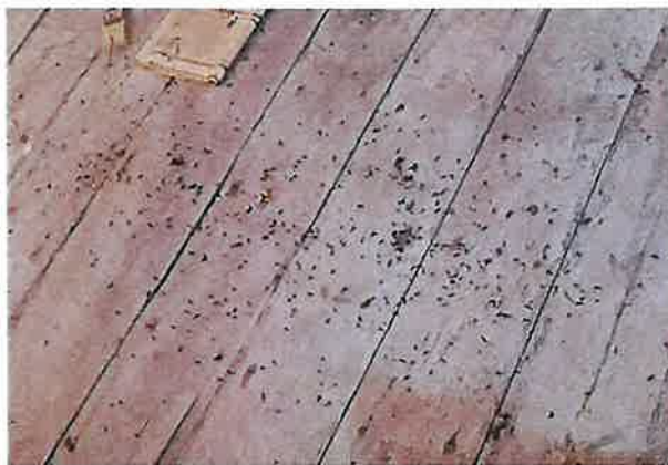
Bat droppings on floor of void
