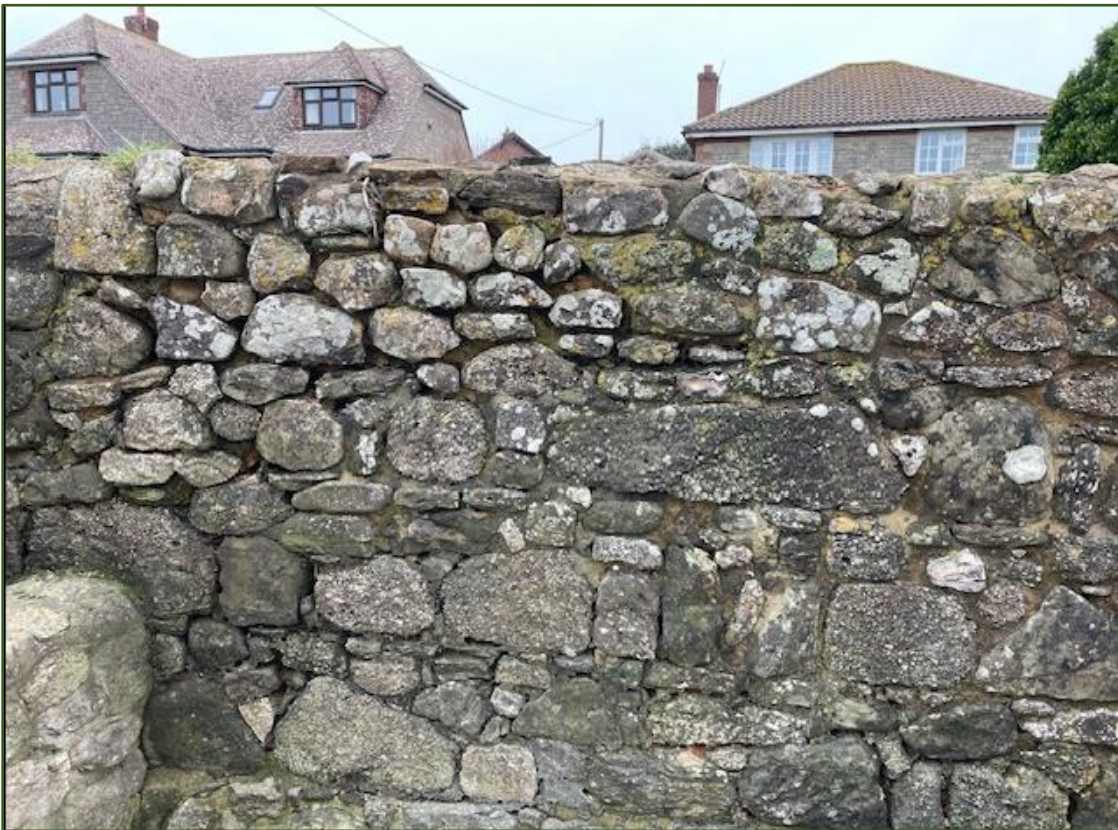
Figure 32. Historic boundary wall of The Old Brewhouse looking north towards C20 development.
