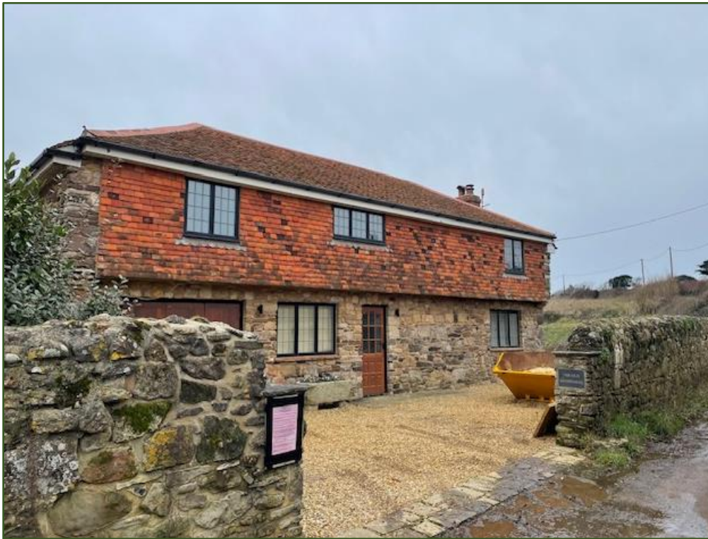
Figure 19. North facing front elevation showing inconsistent size and design of fenestration and inconsistency in style and materials.
