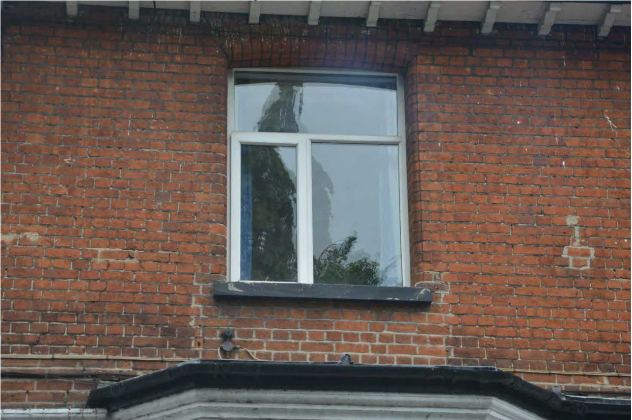
Plate 22: Scars from removal of doors
