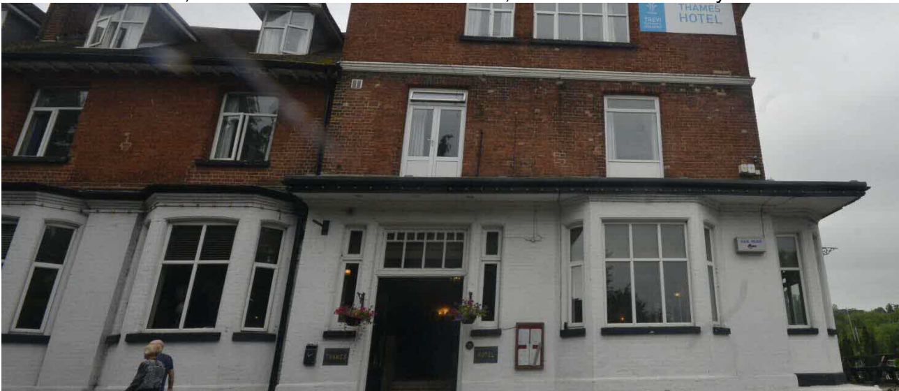
Plate 21: Balcony platform without railings
