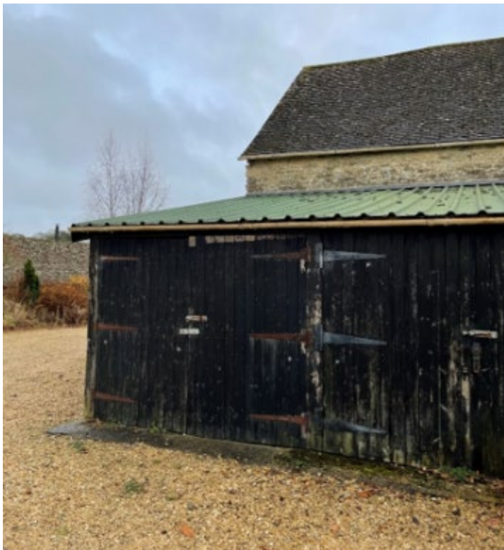
Plate 12: Listed barn, north-west elevation, detail of modern lean-to infilling the northern corner.
