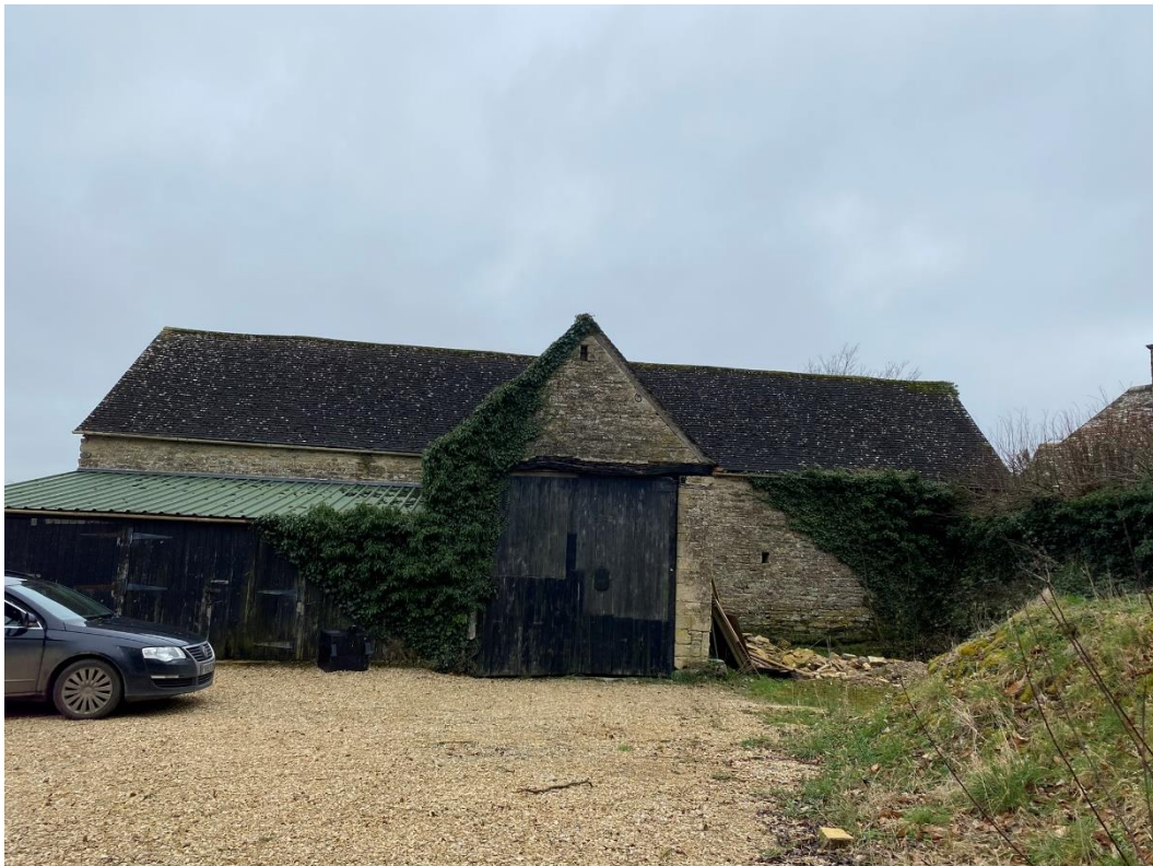
Plate 2: Side (NW elevation) of the barn showing more recent single storey lean-to
