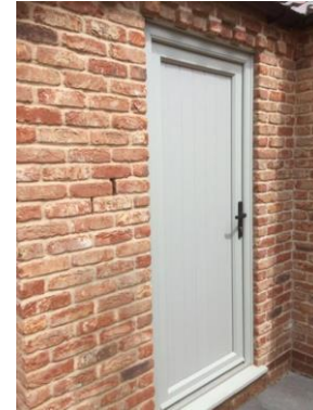
Solid Yeldham door (in white) replacement to the garage (Height and width as per existing)
