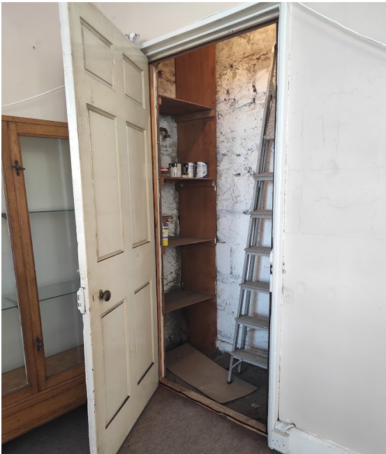
24 First Floor cupboard
