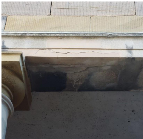
17 Broken stonework to lintels
