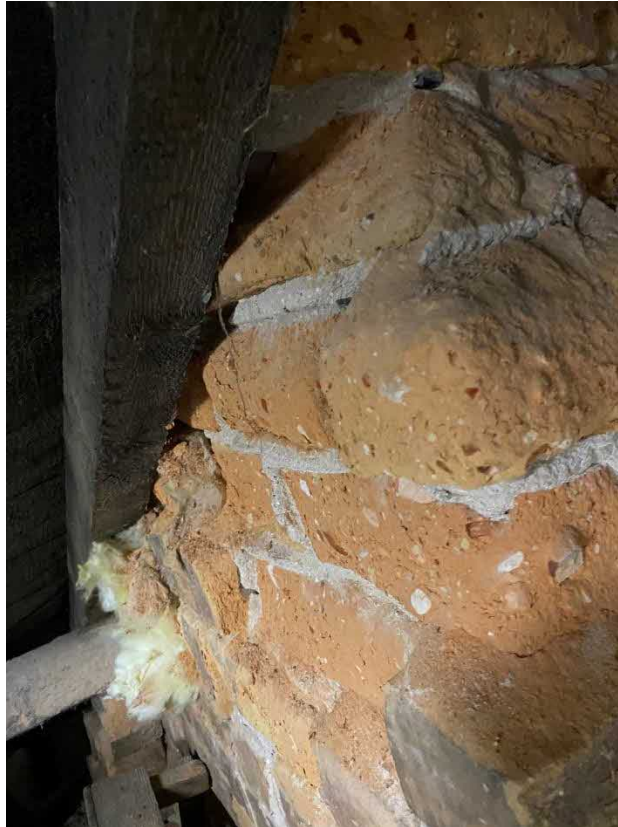
Severely Eroded Brickwork in Roof Space
