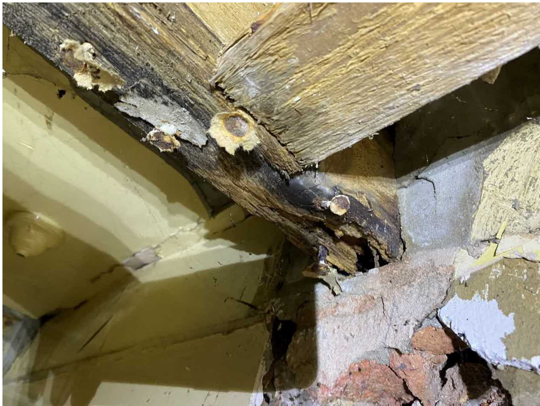
Rotten Timber in Ceiling
