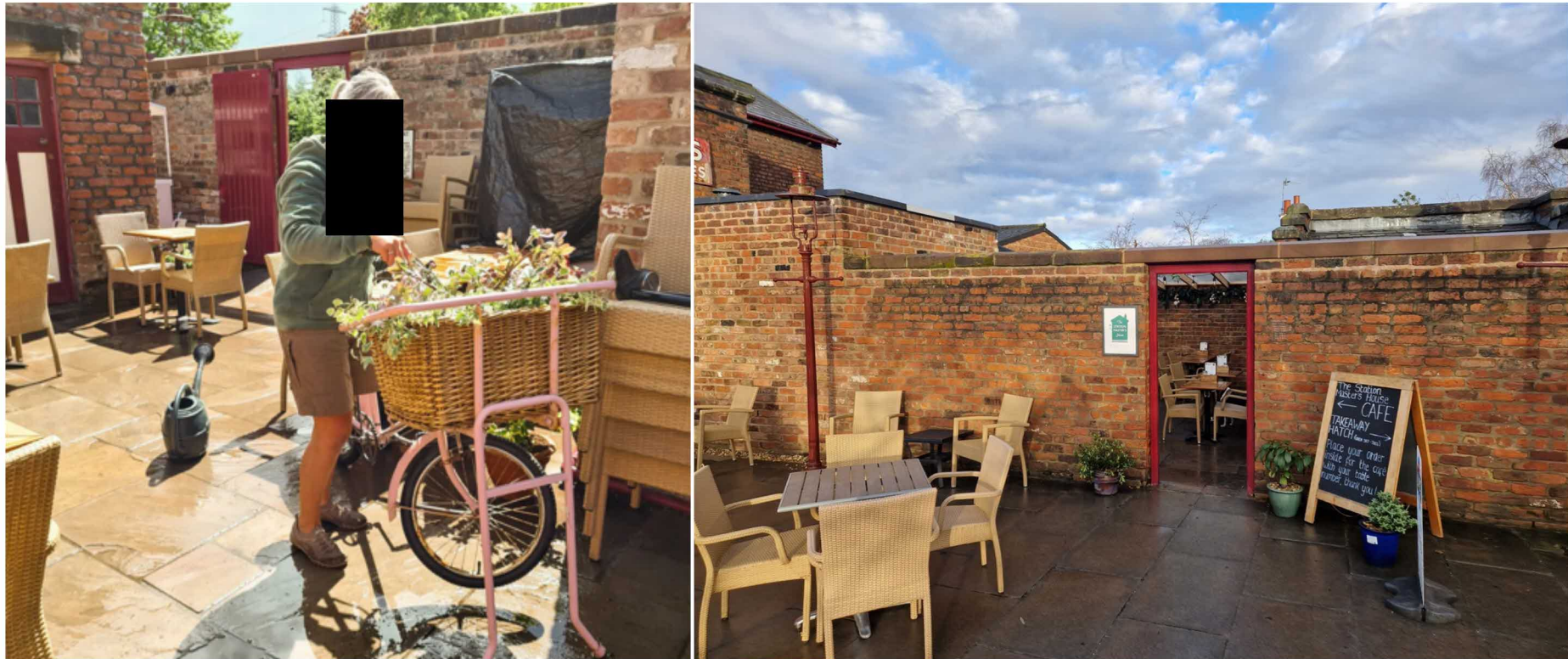
Left: The Courtyard prior to the roof installation; Right: the courtyard with the roof installation as seen from the platform.
