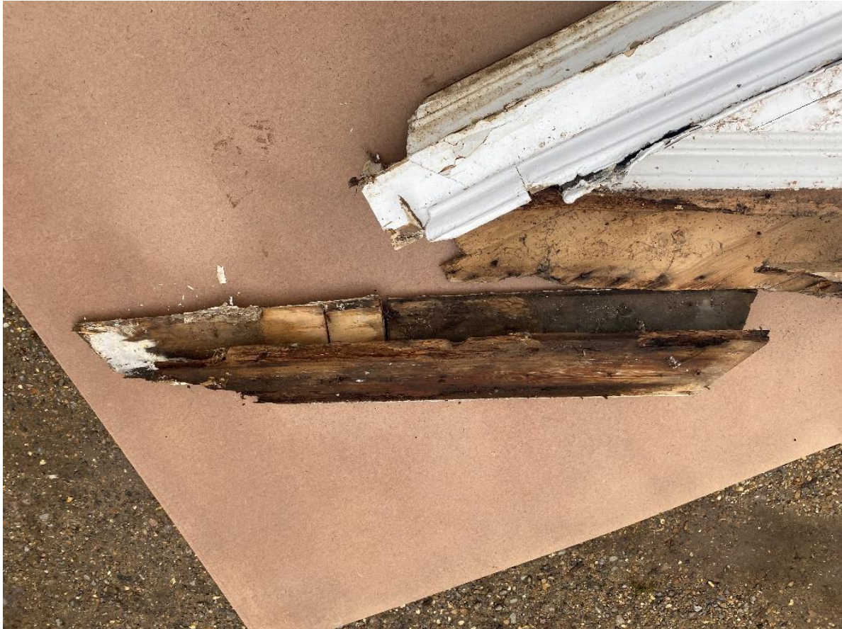
The poor condition of the removed pediment
