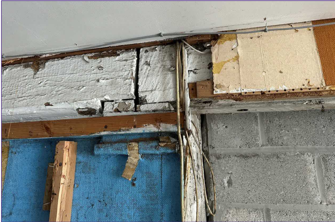
Detail showing but joint between the historic principal beams above the concrete-block spine walls. Before the wall was inserted, there would have been a brick or stone pier at this location. A new pier is included in the proposals.
