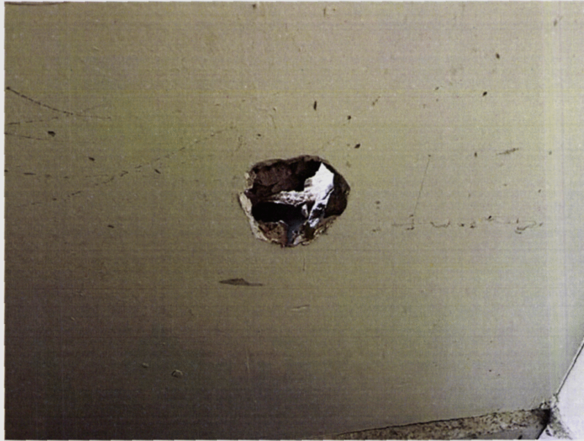
Confirmation that the partitions around office 3 and toilets are all timber stud
