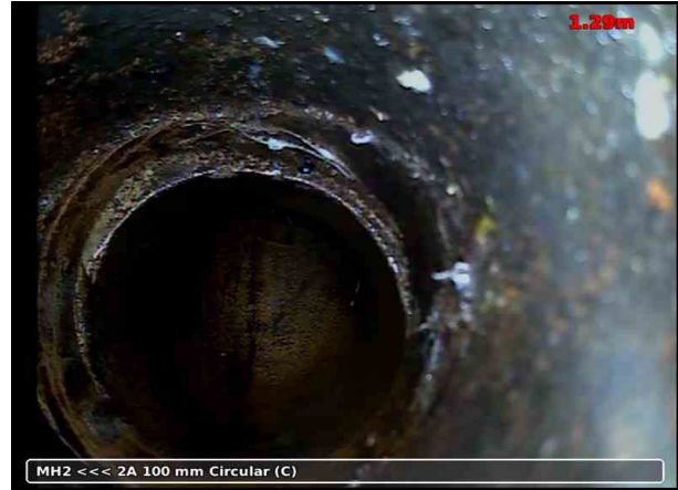
2, 00:00:22, 1.29 m Fracture, circumferential from 12 o'clock to 12 o'clock
