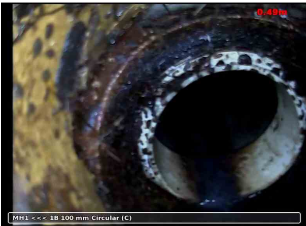
3, 00:00:21, 0.49 m Roots, fine at joint
