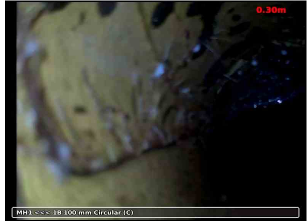
2, 00:00:15, 0.30 m Roots, fine at joint
