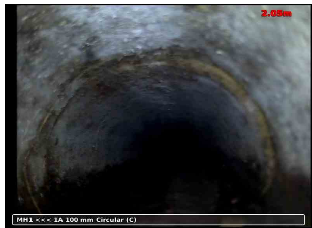
4, 00:00:41, 2.05 m Crack, circumferential from 7 o'clock to 11 o'clock
