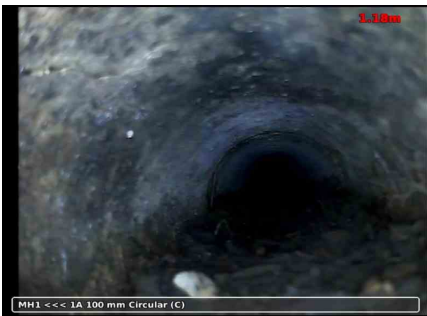
3, 00:00:26, 1.18 m Settled deposits, hard or compacted, 40% cross-sectional area loss, start
