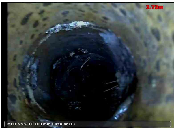
5, 00:00:52, 3.72 m Crack, circumferential at joint from 8 o'clock to 4 o'clock
