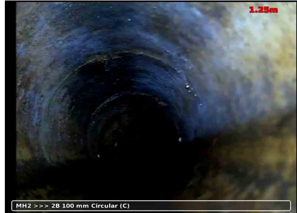
2, 00:00:23, 1.25 m Crack, circumferential from 8 o'clock to 2 o'clock
