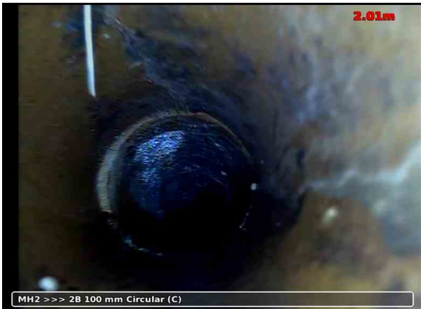
5, 00:00:42, 2.01 m Joint displaced, medium
