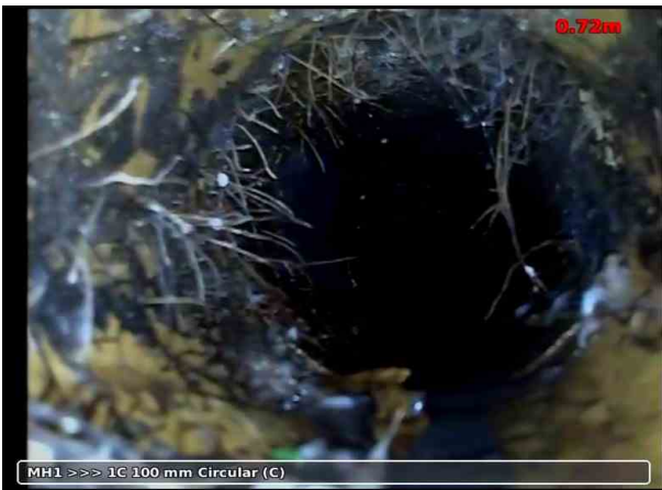
3, 00:00:20, 0.72 m Roots, mass at joint, 10% cross-sectional area loss
