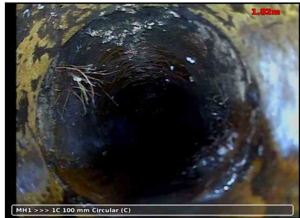
4, 00:00:34, 1.82 m Roots, fine at joint
