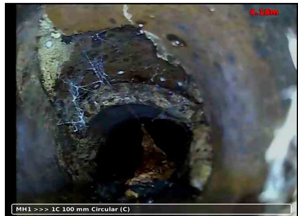
6, 00:00:59, 4.18 m Collapsed drain or sewer
