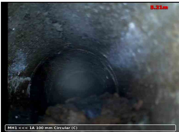
5, 00:01:35, 5.17 m Junction at 9 o'clock, diameter: 100mm
