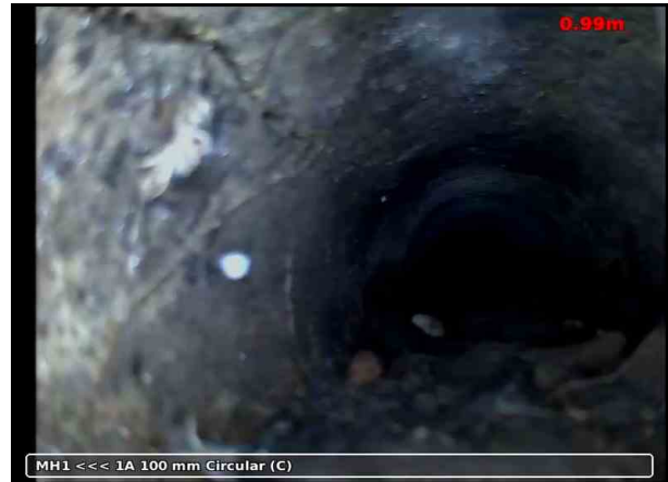
2, 00:00:24, 0.99 m Fracture, longitudinal at 10 o'clock
