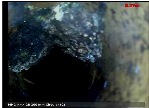
6, 00:01:16, 6.23 m Attached deposits, other at 12 o'clock, 20% cross-sectional area loss, Grease
