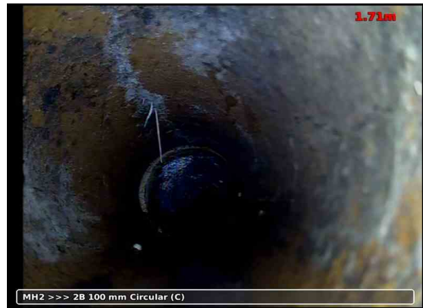
4, 00:00:41, 1.71 m Crack, longitudinal at 11 o'clock, start, Fine root ingress through crack
