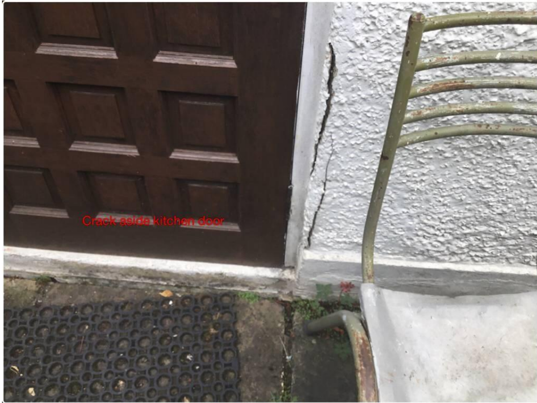
Damage Adjacent to kitchen door - Rear
