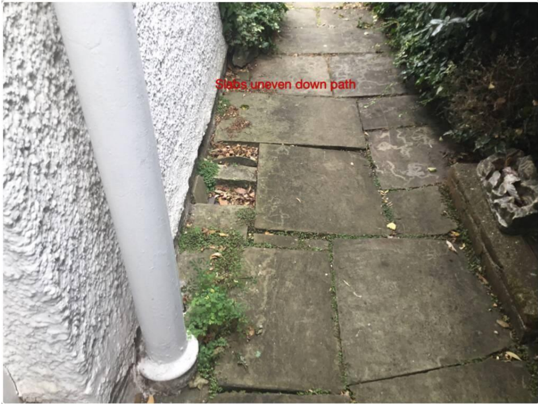
Long term settlement of paving
