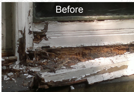
Rotten unsalvageable sill
