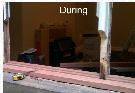
Sill replaced with bespoke new timber and rot cut out from sash frame
