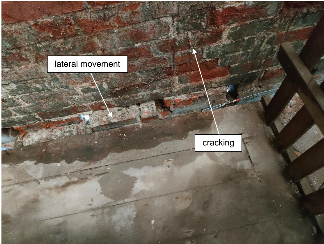
Image 6 Upper floor, lateral movement at floor level.
