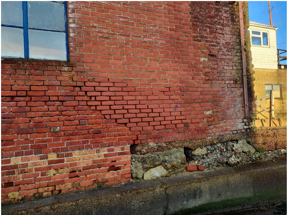
Image 17 Slab, stone and fill support to right hand side elevation wall to rear.
