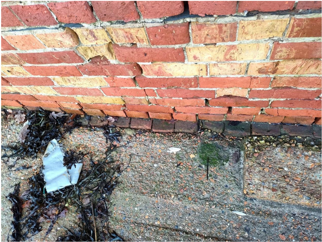
Image 16 Right hand side elevation – spalled brickwork and loss of mortar.
