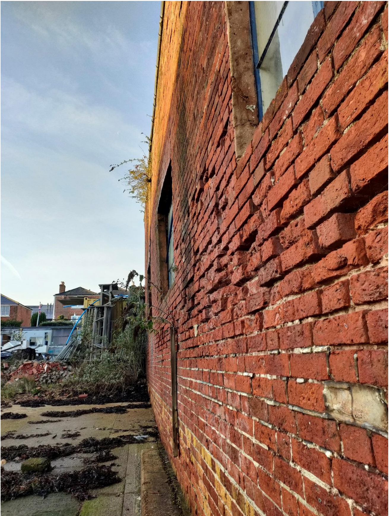
Image 15 View along right hand side elevation showing significant spalling and bow.
