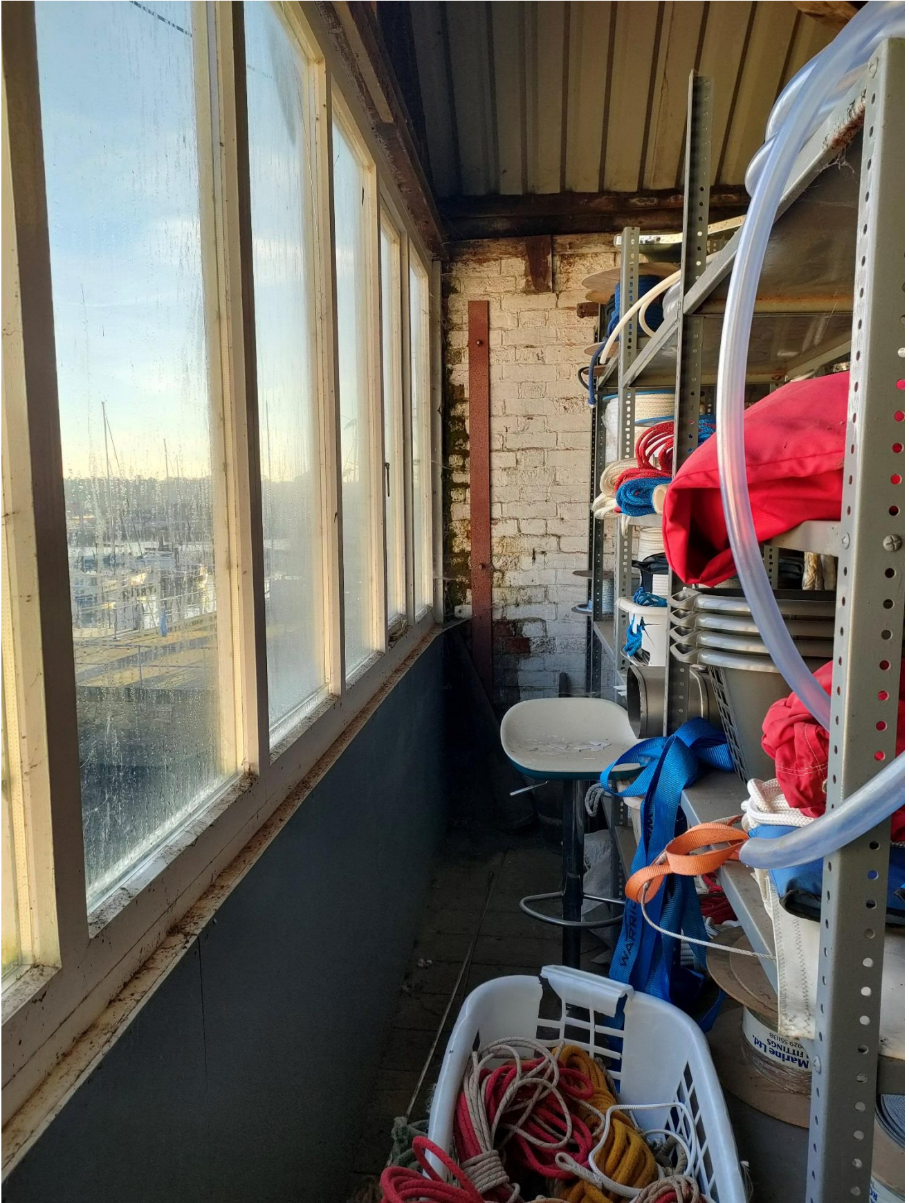
Image 7 Upper floor, rear – steel strapping.
