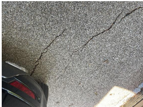
Pictures 3 – Cracking to resin drive
