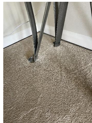
Picture 2: Gap between floor & skirting
