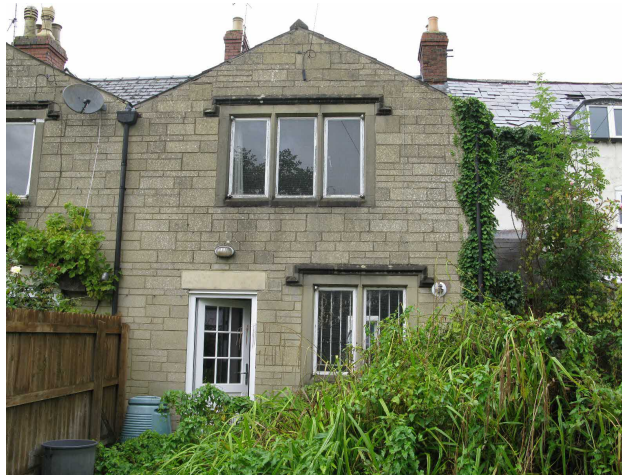
View of rear elevation showing historic stone built rear extension with shared valley gutter at the party wall line.
