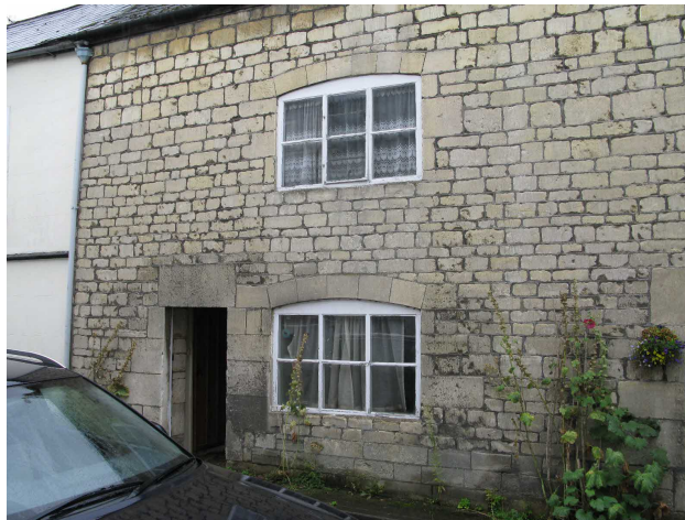
View of existing Front elevation showing the segmented arched headers to the windows, and deep lintel over the entrance all in hammered Cotswold stone.
