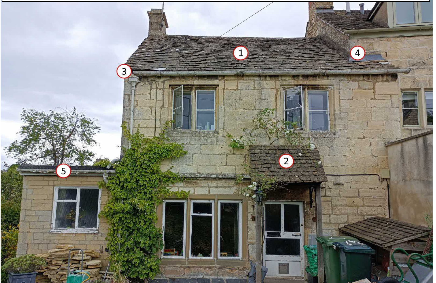
Eastern Building Elevation – Numbering refers to the 'Feature No.' contained in Table A3-1 within Appendix 03
